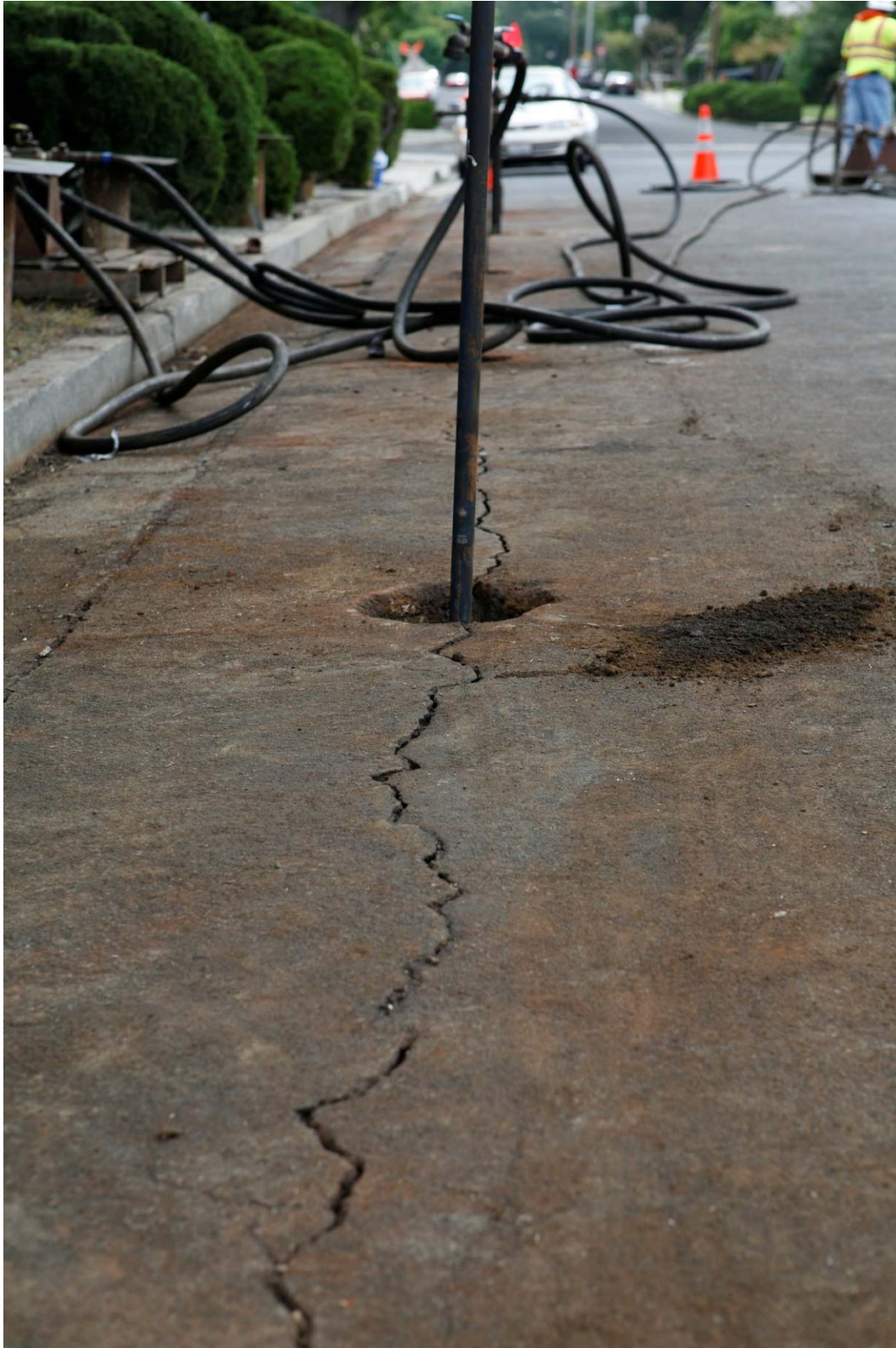
Figure 15. Demonstration of Fracture Along Alignment of PRB
