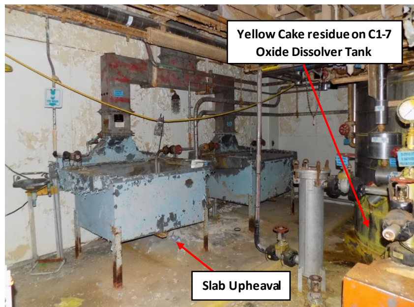
Photo 03: This image shows the decontamination sink on the left and the rinse sink on the right on the first floor in Zone 5.1.2, Room 103. The photo shows an upheaval of the slab on grade concrete beneath them. There appears to be no additional upheaval since the previous S&M Inspection in 2020. This is not a structural or a personnel safety concern since it is a slab on grade and the area is protected by a rope barricade with warning signs. The C1-7 Oxide Dissolver Tank located right of the sinks shows yellow cake residue. Residue has not increased since the previous S&M Inspection in 2020.
