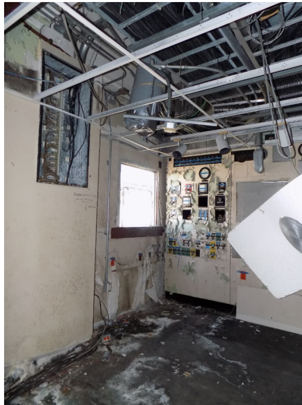
Photo 07: The photo above shows the general condition in Room 206, Zone 5.2.1. It shows an example of the amount of mold present on the walls and floor. The window could have been the source of the moisture causing the mold. There appears to be no additional mold growth in the area since the previous S&M Inspection in 2020.
