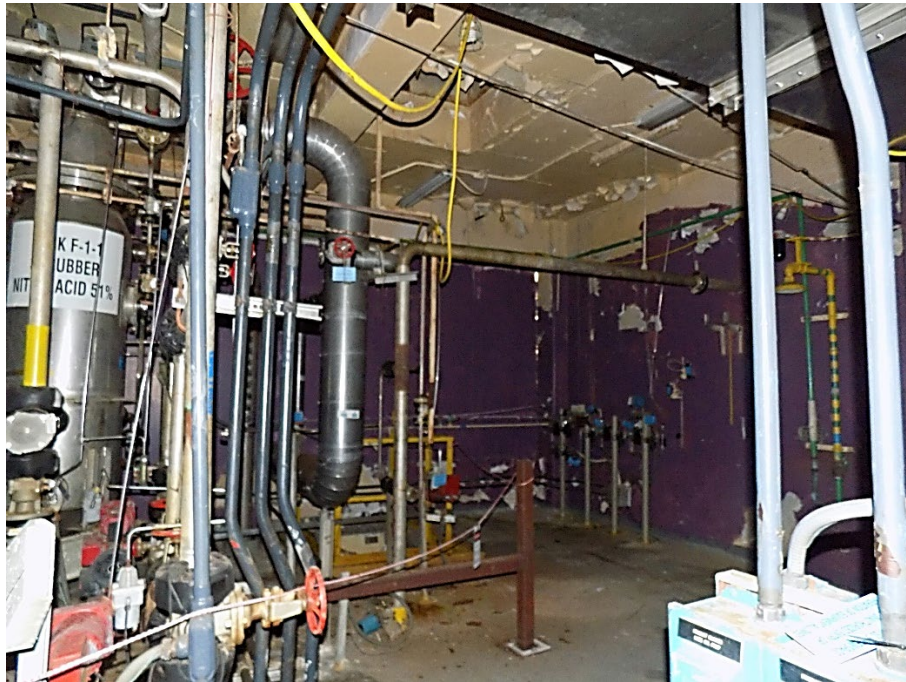
Photo 12: The above photo shows a typical example of the deterioration on the coating for fixed contamination on the third floor in Room 302, Zone 5.3.2. The deterioration does not appear to have worsened since the previous S&M Inspection in 2020.
