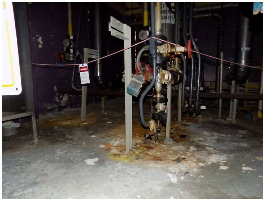
Photo 11: This photo shows a view of the acid spill on the third floor in the area of the Venturi Scrubber, F-1-1 (Room 302, Zone 5.3.2). The area is protected by a rope barricade with warning signs. There appears to be no additional degradation since the previous S&M Inspection in 2020.
