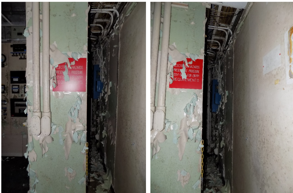
Photo 09: The photos above show the area behind the control panel in Room 207, Zone 5.2.1 (Control Room) and the extent of the peeling paint in that area. This condition is judged to be non-structural in nature.
