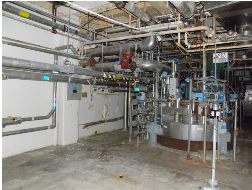
Photo 02: This image shows the general condition of the Denitrator Reactors located on the first floor in Zone 5.0, Room 104. There appears to be no change since the previous S&M Inspection in 2020.
