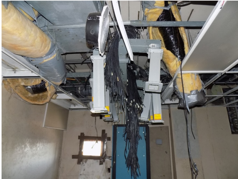
Photo 08: The photo above shows the condition of the ceiling in Room 206, Zone 5.2.1. The hanging wires were discovered during the 2020 S&M Inspection. There appears to be no additional deterioration of the ceiling since the previous S&M Inspection in 2020.
