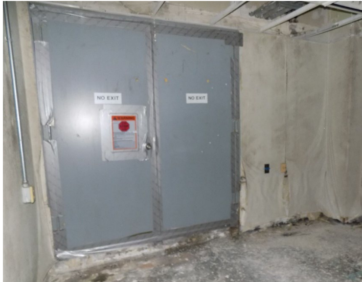
Photo 06: The photo above shows the exit doors on the north end of the second floor of A-Line. The tape around the door edges is secure and the “No Exit” signs are clearly posted.
