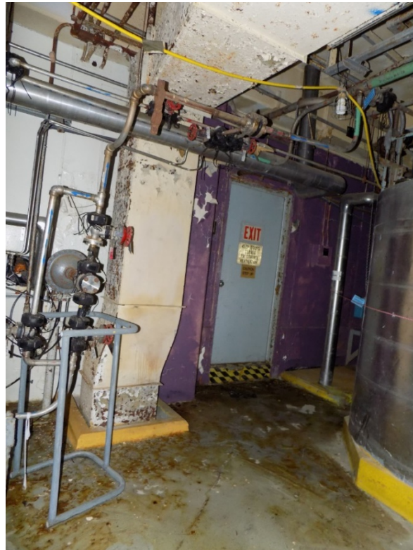
Photo 04: The above photo shows the typical condition of the concrete floor on the second floor in Zone 5.2.2, Room 208. There is moisture on the floor with the source appearing to be from the doorway. The moisture has caused staining on the floor. There appears to be no additional staining or degradation of the concrete since the previous S&M Inspection in 2020.
