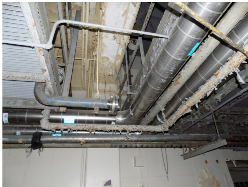
Photo 05: The photo above is a typical example of the deterioration of the paint coating around the pipes and the paint on the ceilings on the first floor.
