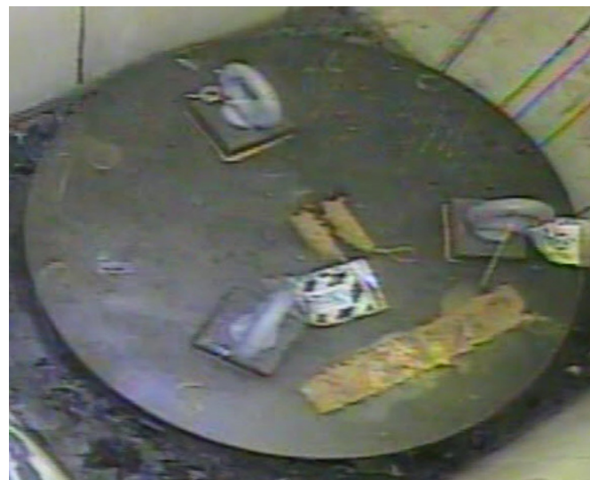
After (With Temporary Riser Cover)
