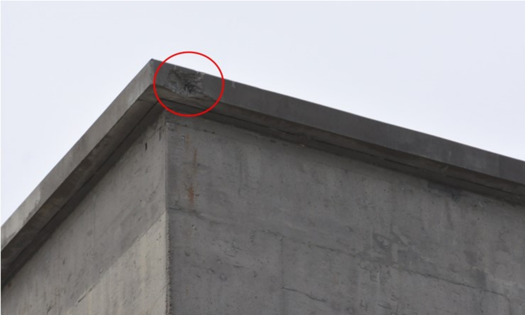
Figure O-6. View of 105-P Actuator Tower Roof Cap Flaw (2017)
