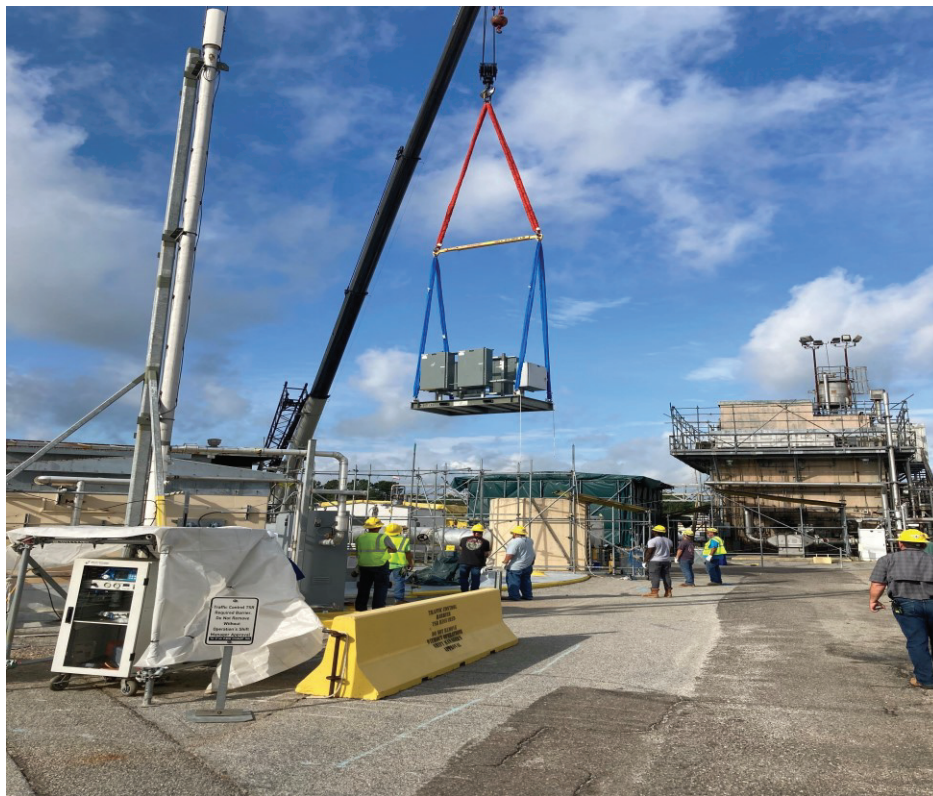
Figure 6: Tank 27 CSMP Contactor Skid
