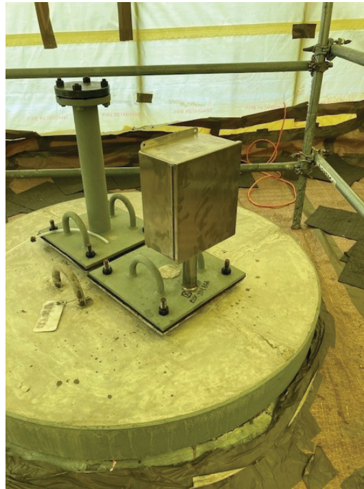
Figure 10: Tank 39H High Liquid Level Conductivity Probe (HLLCP) Junction Box
