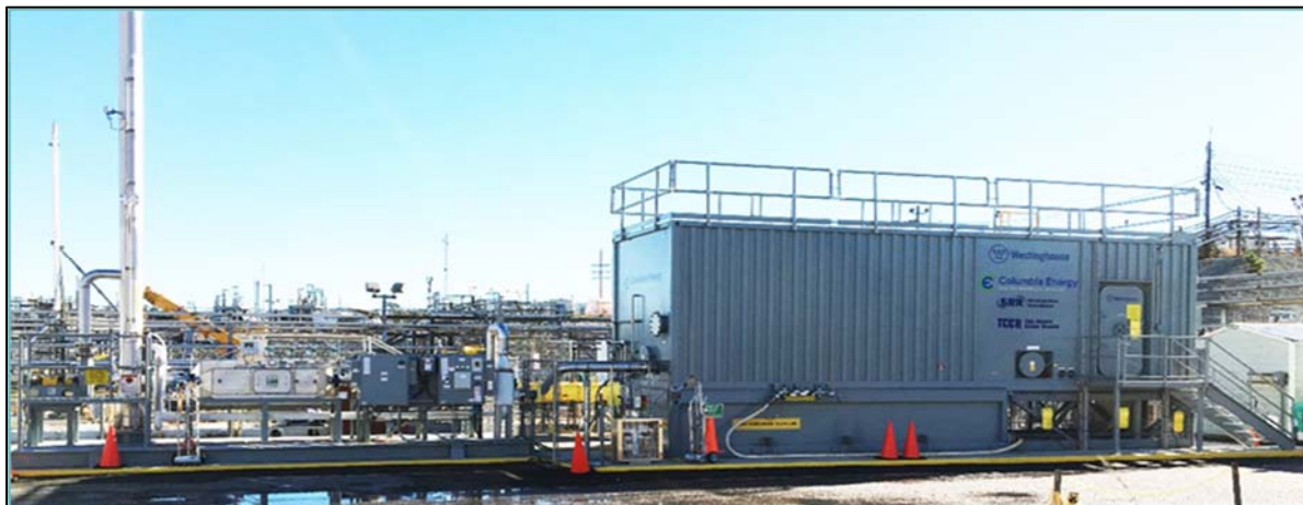
Figure 1: TCCR Process Enclosure and Ventilation Equipment
