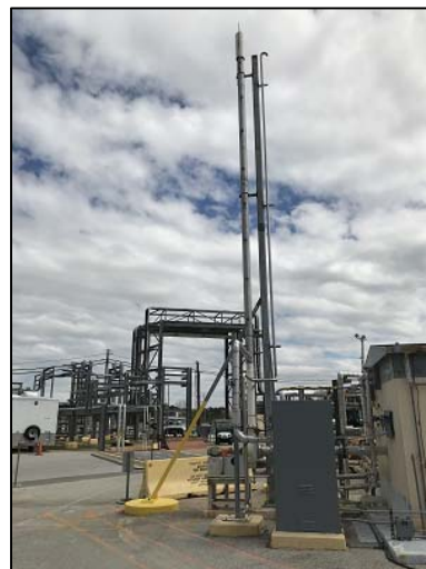
Figure 6: Tank 27F Exhaust Stack Extension
