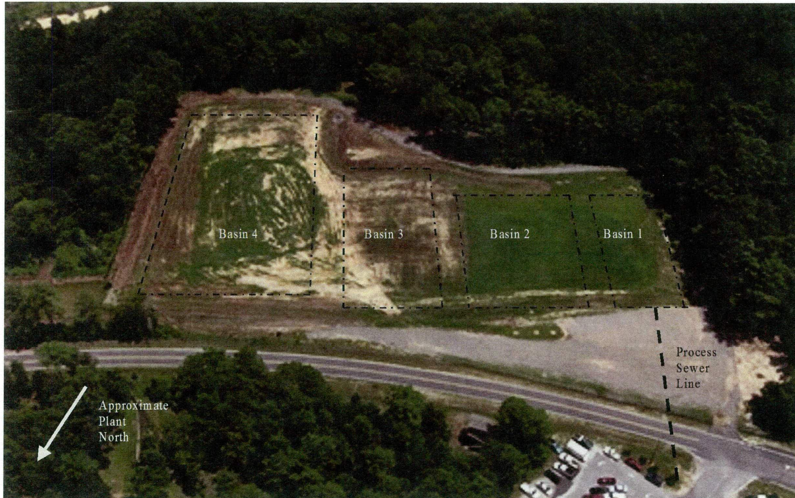
Figure L-2. Layout of the SRLSB OU (904-53G, 904-53G, 904-54G, and 904-55G) after Construction Completion August 2001
