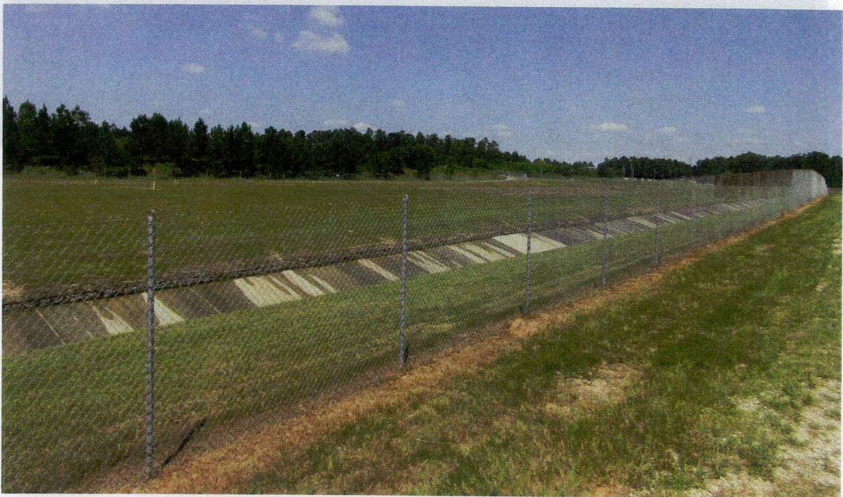
Figure G-4. Current On-Unit Photographs of the Cover System of the HHWMF OU (2016)
