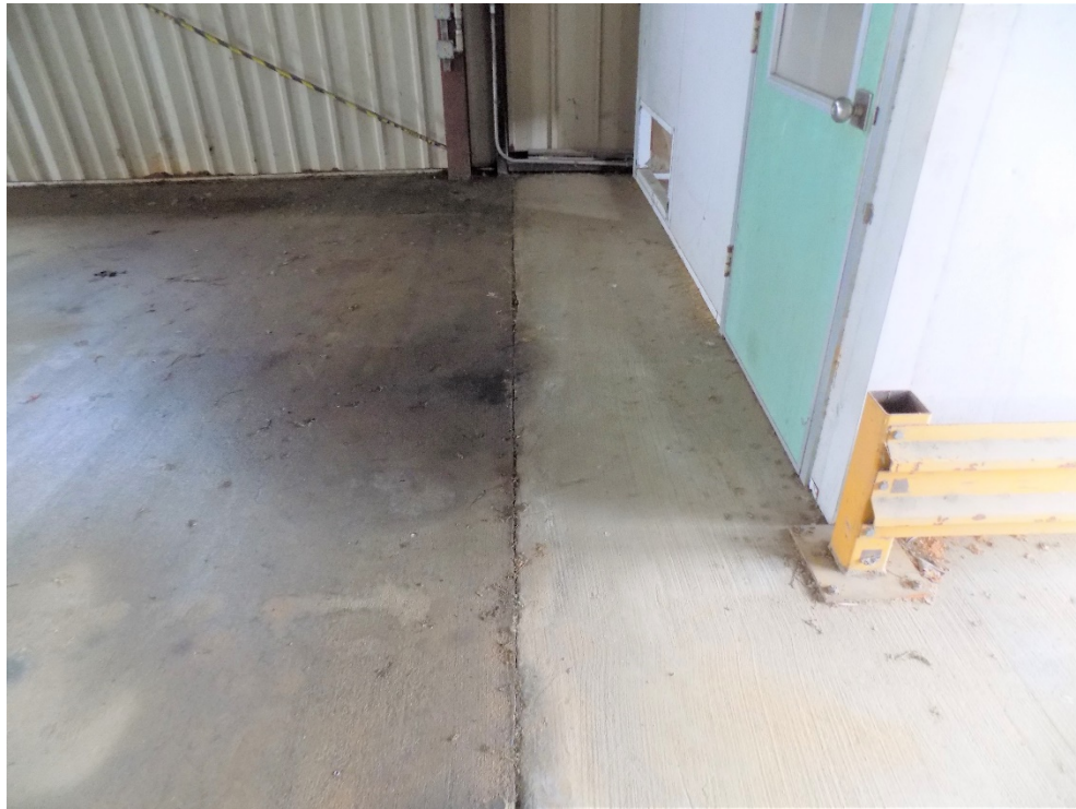
Figure 6. Building 484-13D, D-Area Storage Building Floor Stain
