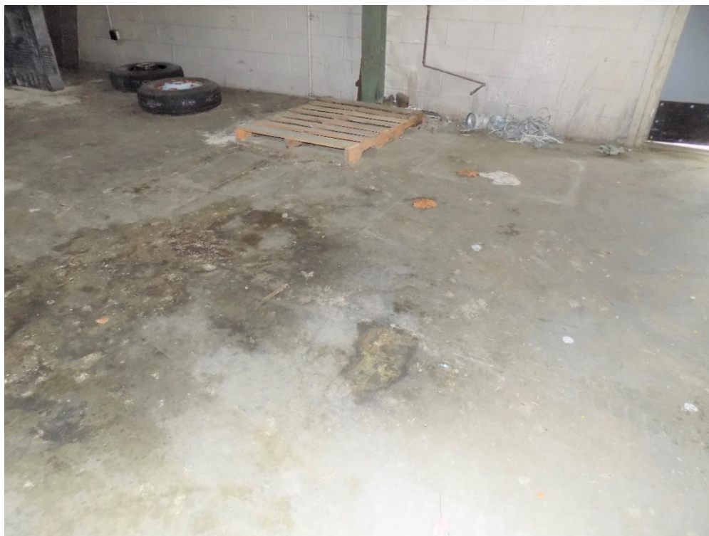
Figure 1. Stained Concrete Near East Door
