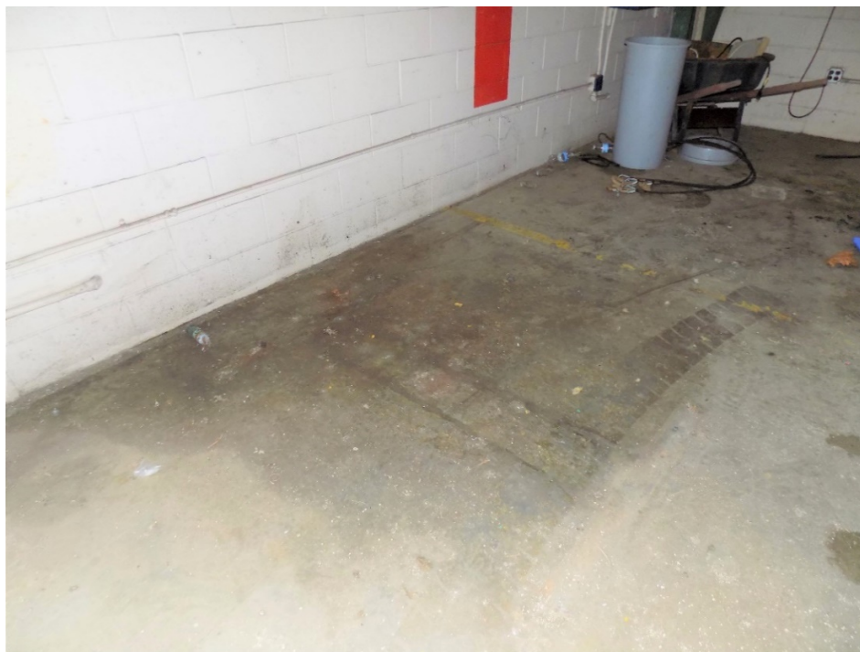
Figure 2. Stained Concrete Near Wall Perpendicular to South Wall
