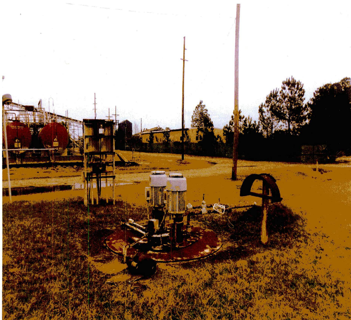
Figure 13. Sanitary Sewage Lift Station 607-12D (currently abandoned)
