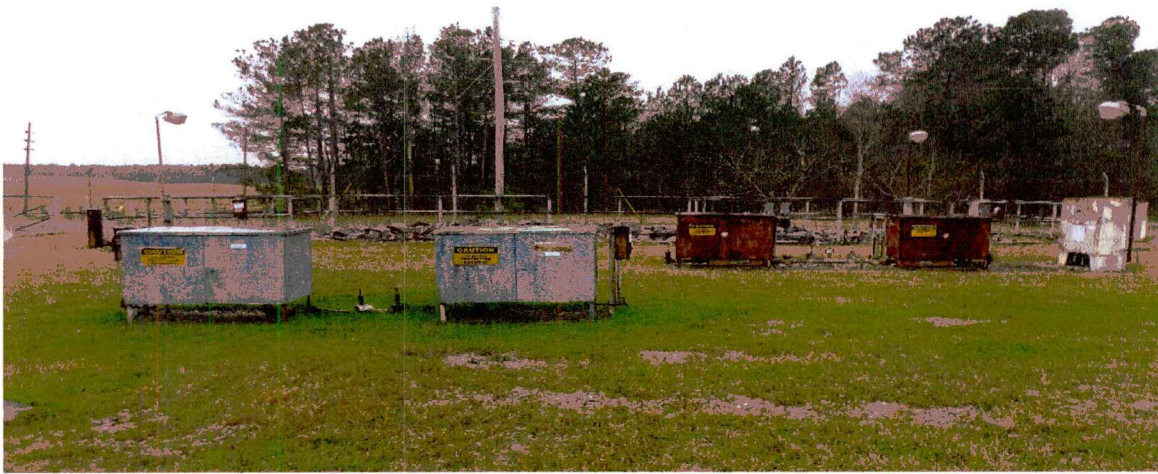
Figure 11. 607-15D Sanitary Treatment Blowers
