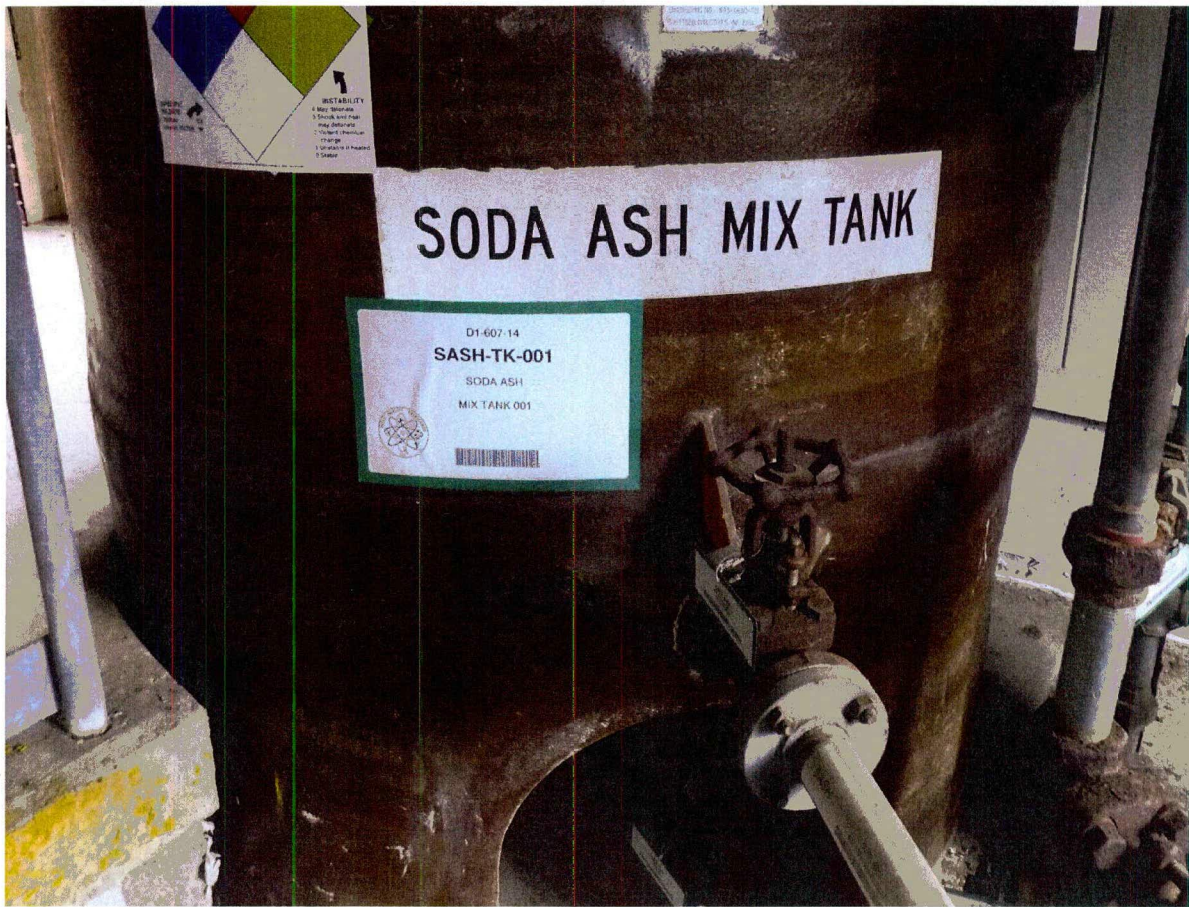
Figure 6. Soda Ash Mixing Tank (607-14D)
