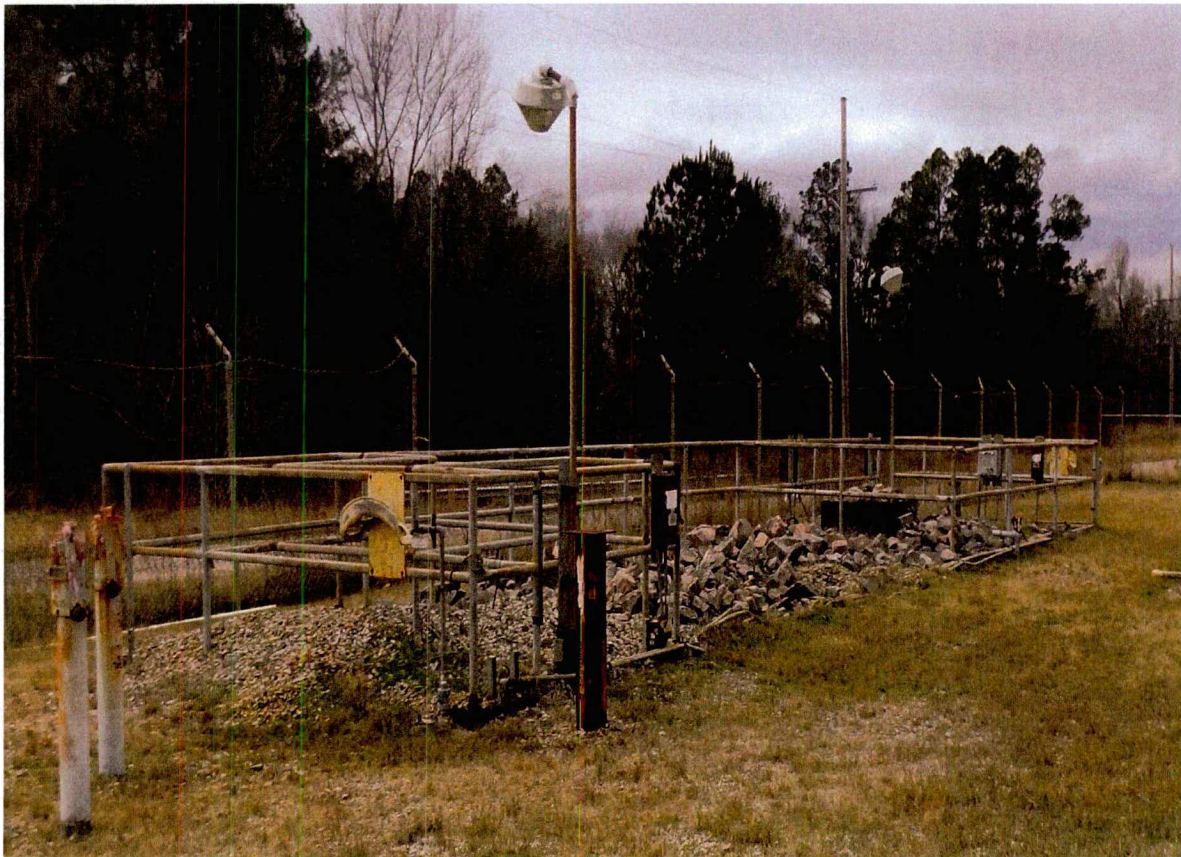
Figure 9. 607-15D, Sanitary Waste Treatment Plant
