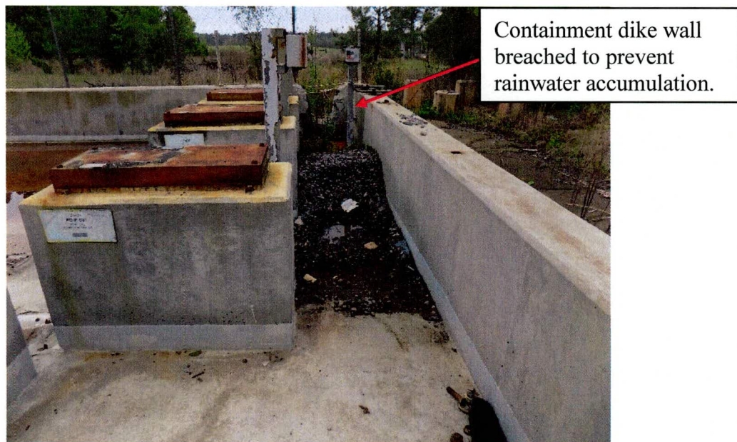
Figure 5. Building 454-D Slab and Sump (Looking West) After Partial Decommissioning by CRO
