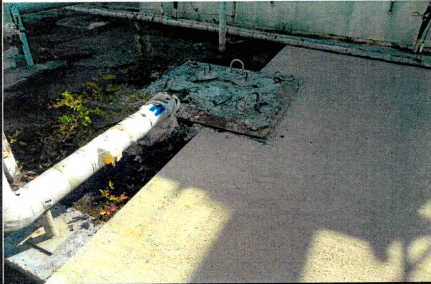
Tank 12, Center Riser
