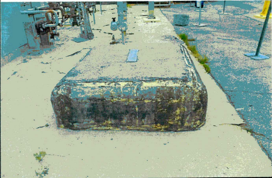
Tank 6, East Annulus Riser
