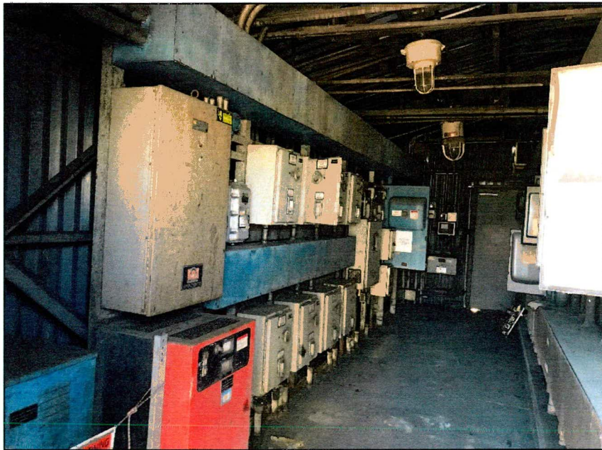
Photograph 2. View of panel boxes inside electrical room (H02 components inside).
