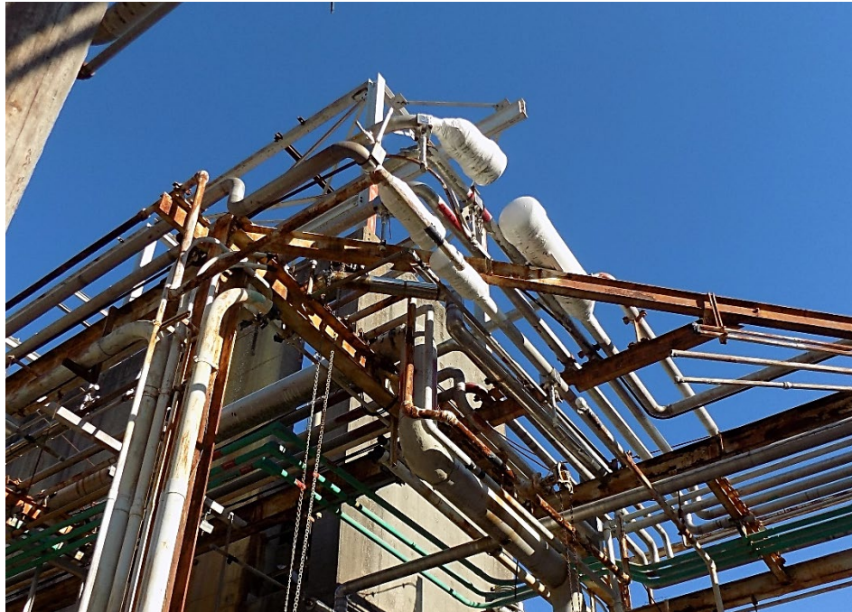
Photo 5 - Pipe Caps/Wraps and Pipe Taps
