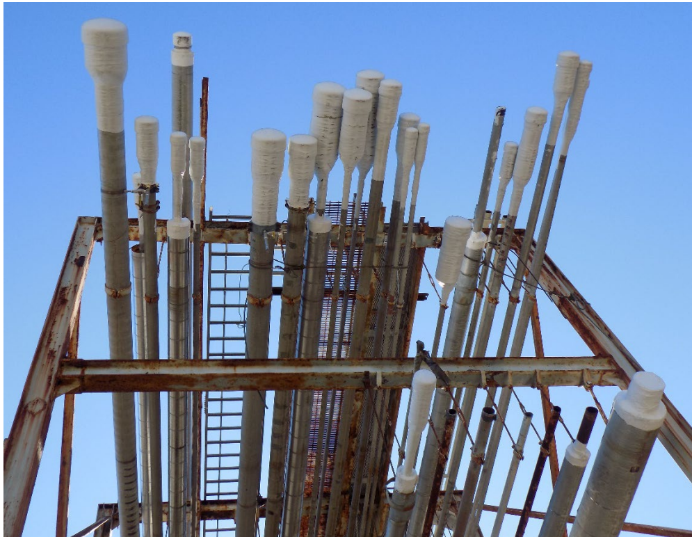
Photo 8 - Pipe Caps/Wraps and Pipe Taps
