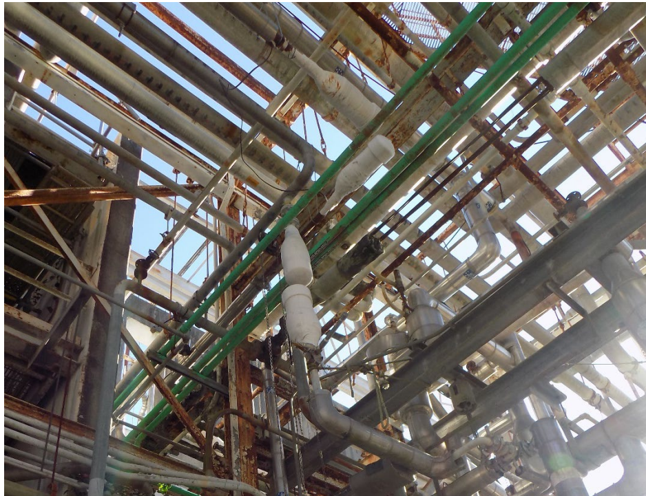
Photo 6 - Pipe Caps/Wraps and Pipe Taps
