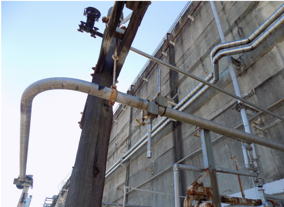
Photo 10 - Pipe Tap Only
