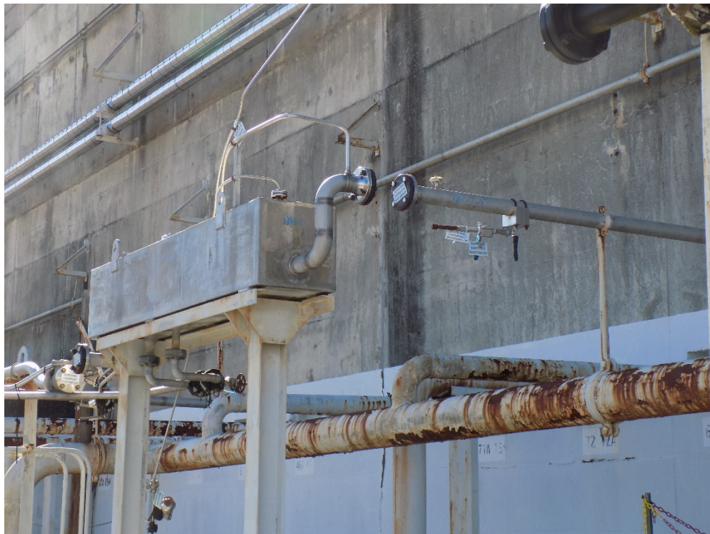
Photo 11 - Pipe Tap Only
