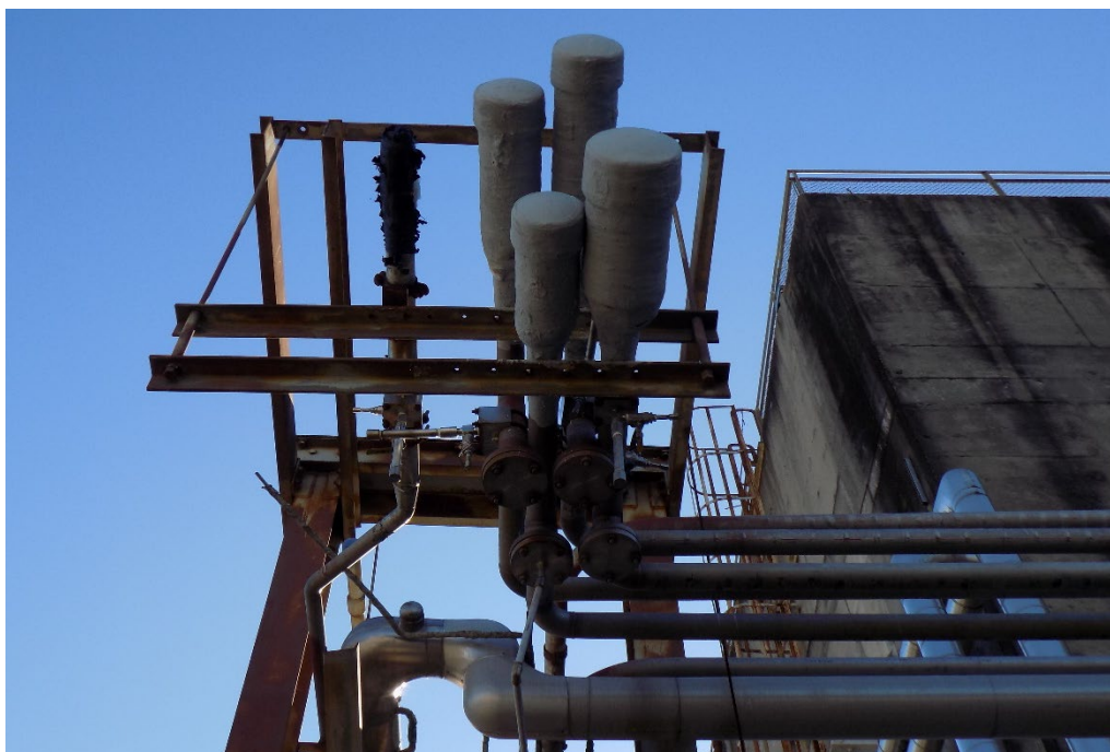
Photo 9 - Pipe Caps/Wraps and Pipe Taps
