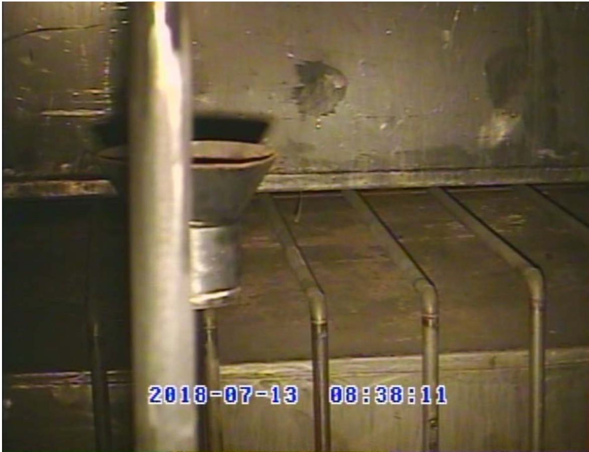
Opening of Flush Water Valve Pit free of accumulated solids
