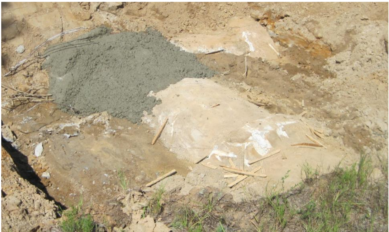
Photo 38. 489-D CPRB Plugged 48" Pipe
