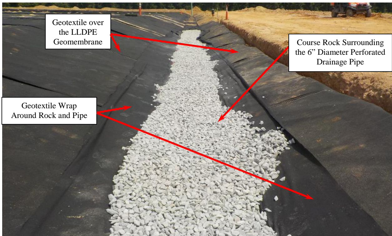
Photo 86. Subsurface Drainage Collection System
