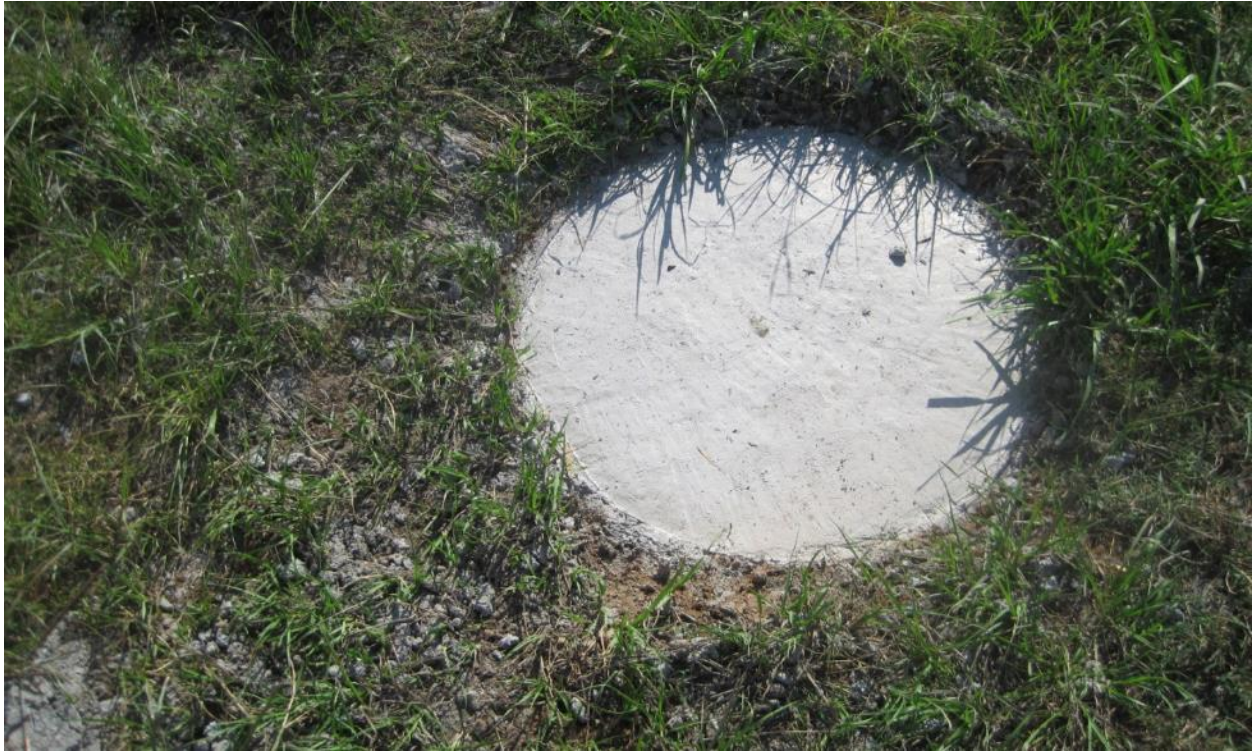
Photo 37. 489-D CPRB Plugged Manhole (Typical for 2)
