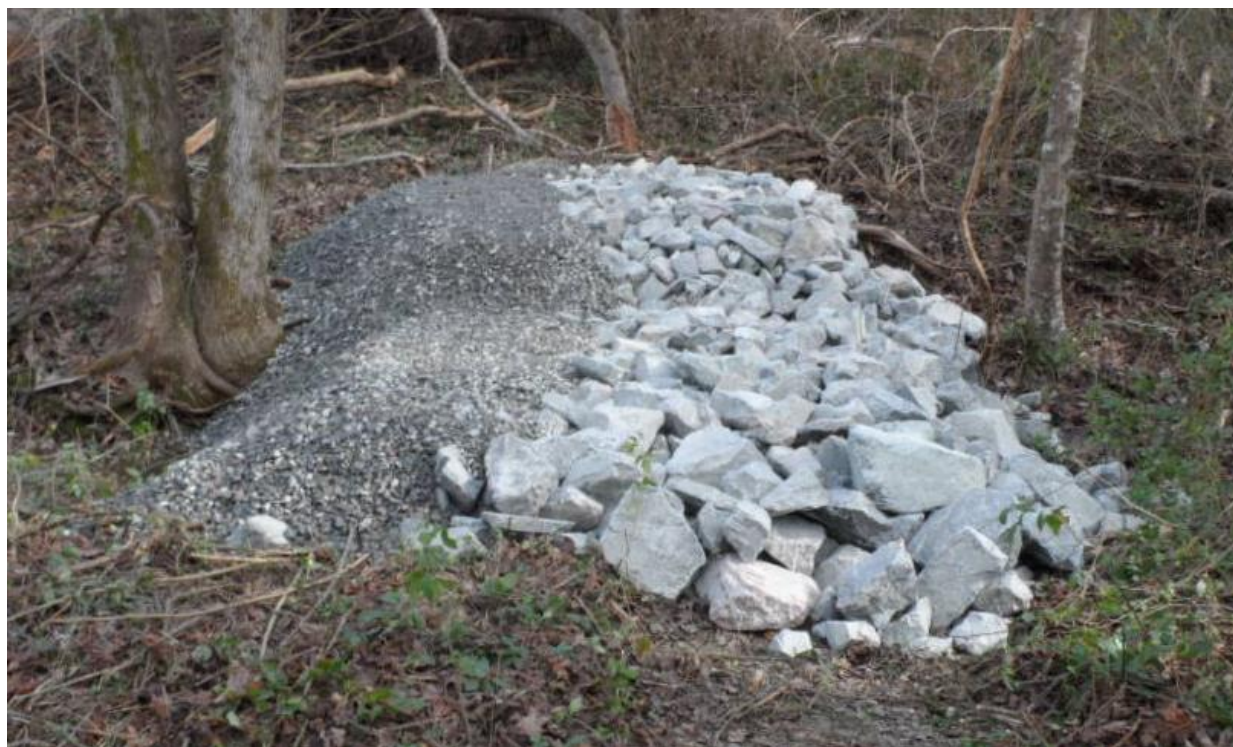
Photo 22. Typical Rock Check Dam
