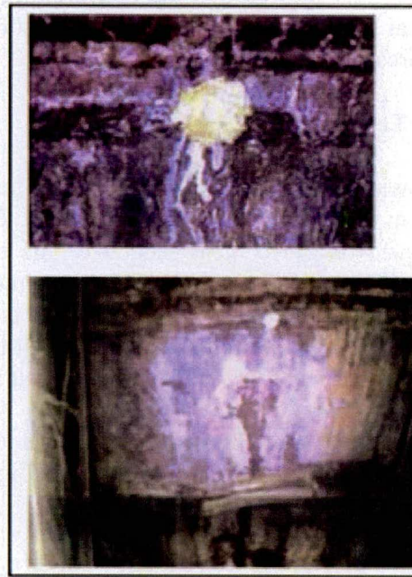
Figure 7: Salt Nodule from North Leak Site
