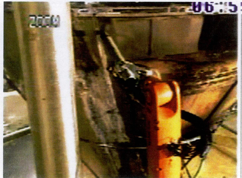
Picture taken during removal of the stainless steel-wrapped insulation on the cone of the evaporator pot
