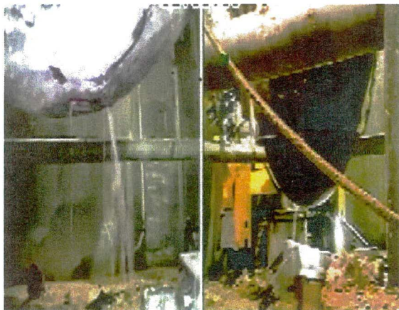
Original Leak Sites
