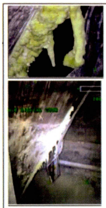
Figure 5: Salt Streak from South Leak Site
