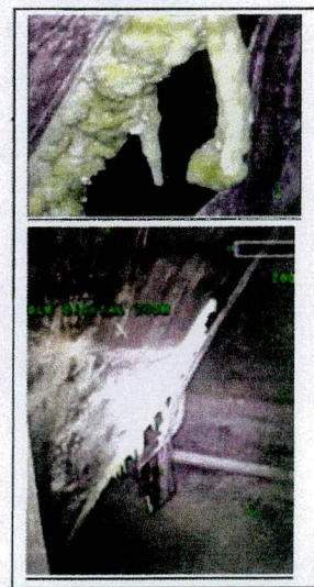
South Leak-site (the salt streak)
