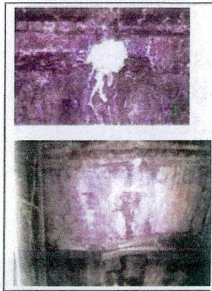
North Leak-site (the nodule)
