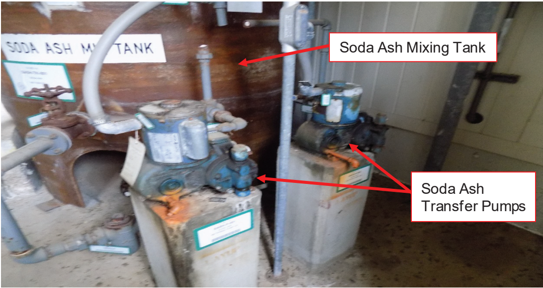
Figure 5. Soda Ash Transfer Pumps/Pedestals (607-14D)
