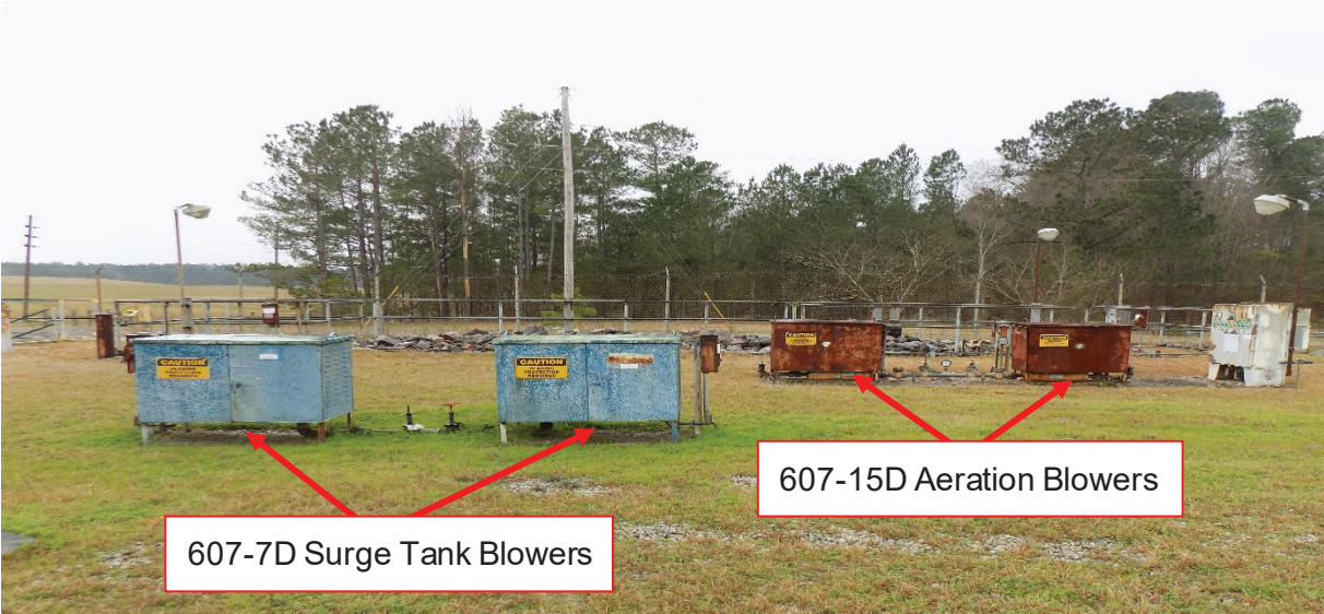
Figure 9. Building 607-15D Blowers
