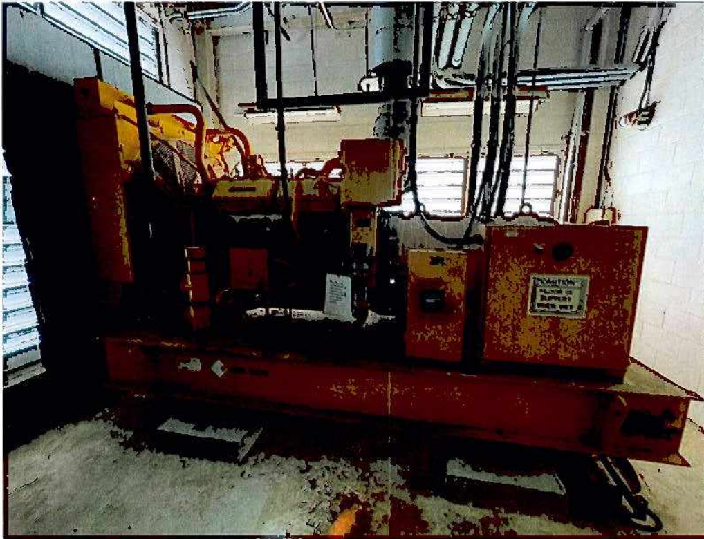
Figure 4: Diesel Generator within 720-F.
