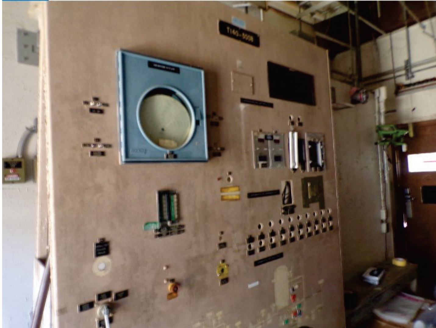
Figure 5. Control Room Panel Post Deactivation
