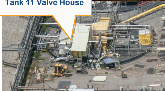
Tank 11 Valve House
