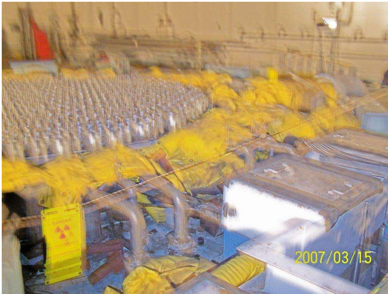
Figure CR-1. Process Area lead in photo taken during maintenance activities in March 2007 (Specific Comment #1)
