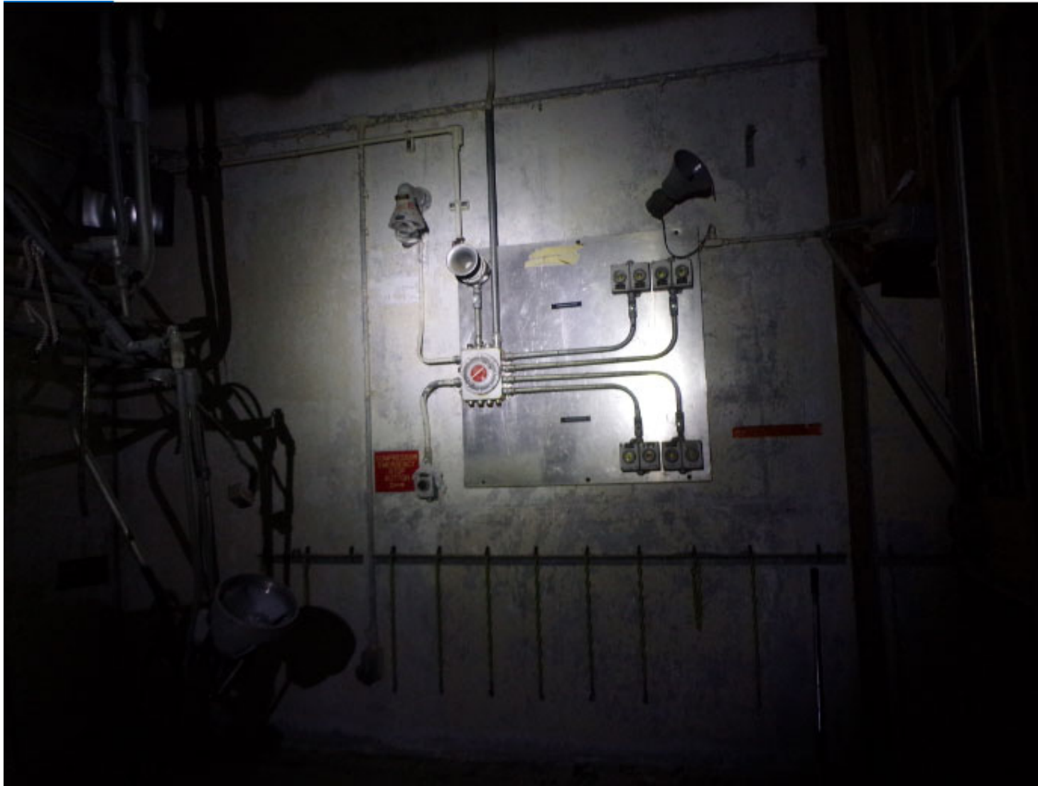
Figure 7. Alarm Panel Post Deactivation
