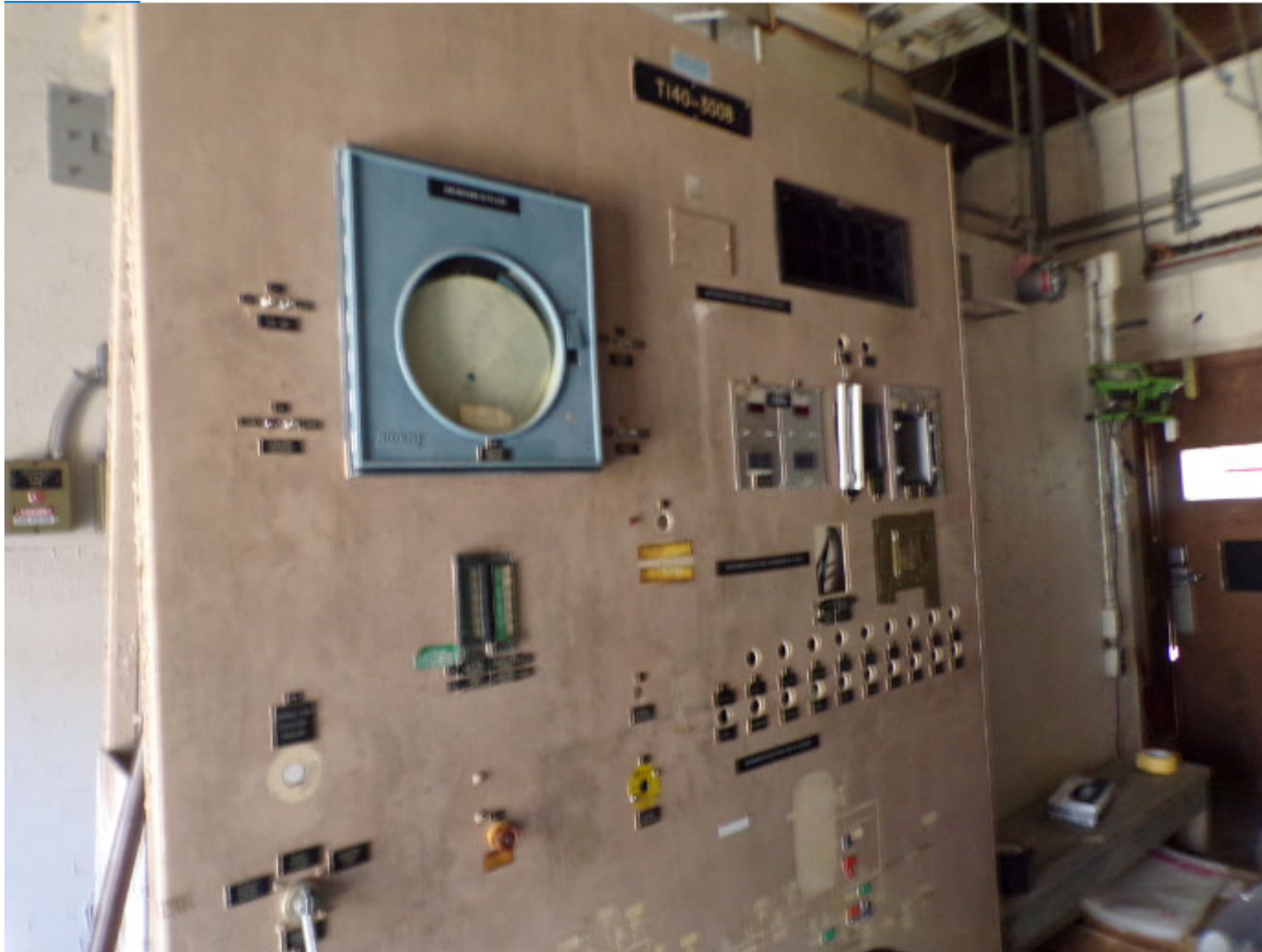
Figure 5. Control Room Panel Post Deactivation
